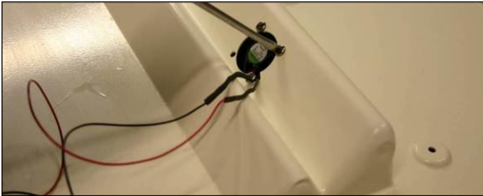
Figure 20a: Evaporator fans
