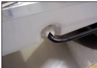
Figure 21a: Drain pipe and putty
